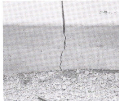
Typical crack at a contraction joint
